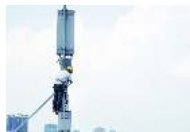
Communication base station
